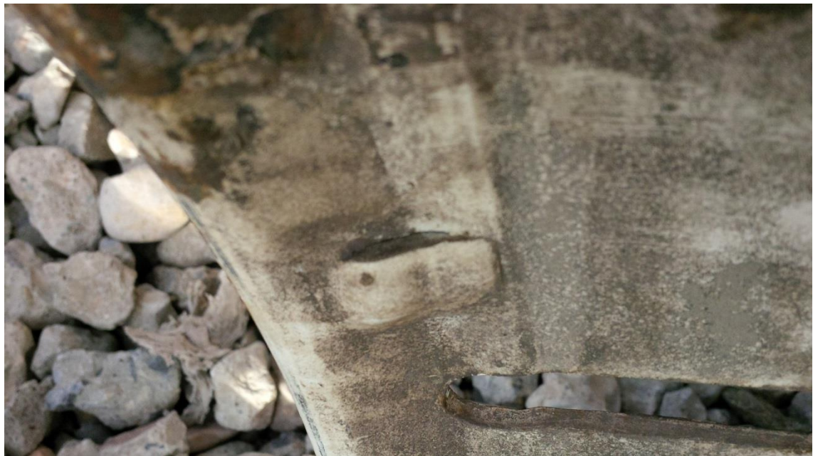
Even though light can be seen between the raised portion of the stop and the rim base, this is not damage
